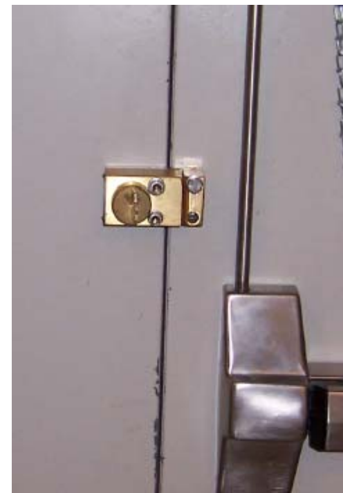
Elevator Stairwell exit door with Kirk Key in Lock
