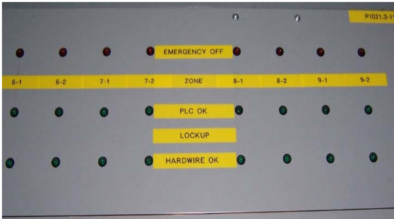
Booster Ring/ Storage Ring ACIS Status Display Panel
